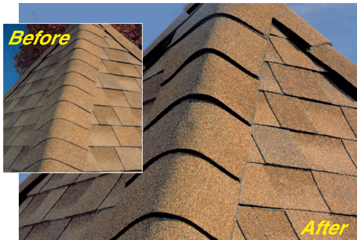
Before: Roof with cut-up strip shingles instead of Timbertex®
