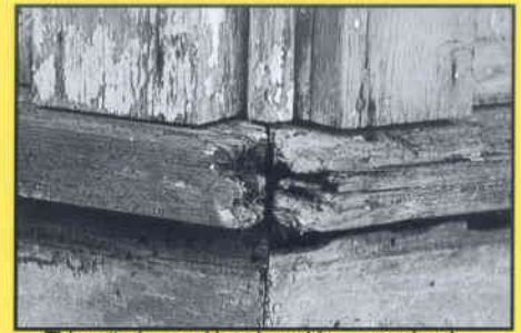
This rotted — and irreplaceable — woodwork ...
