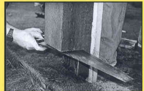
10" rotted bottoms of these load-bearing columns ...
